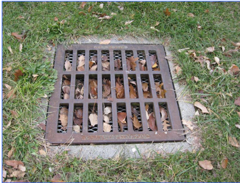
Figure 36: Catch basin with smaller grate size to catch leaves. Catch basins have varying grate sizes. Some jurisdictions use grates with smaller holes or catch basin inserts to trap smaller debris. The drawback is they require cleaning more often for efficiency. 36
