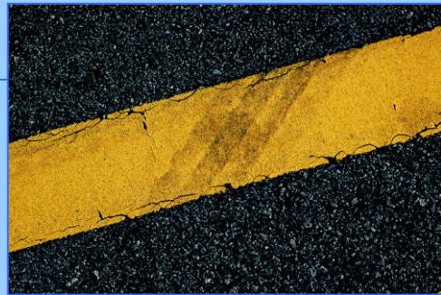
Figure 26: A yellow road stripe. Road striping is necessary for driving, but to protect stormwater, striping should only be performed on clear days with little wind. 26
